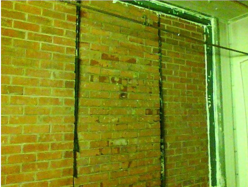
Plate 1 - Safeguard Wall on Completion of 25 Years Accelerated Weathering (STORMDRY Masonry Coating LHS/Control Centre/Trial Product X116 Masonry Coating RHS)
