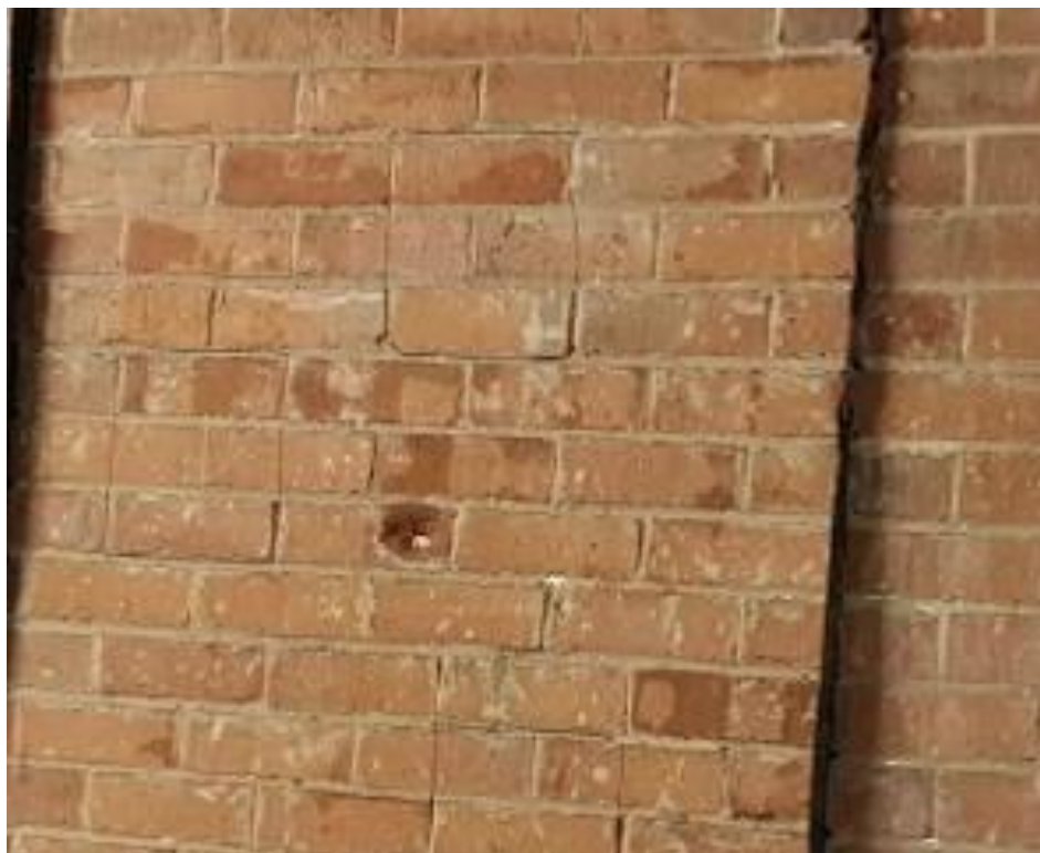
Plate 4 - Front Face of Wall with the Uncoated Bricks showing Signs of Frost Damage
